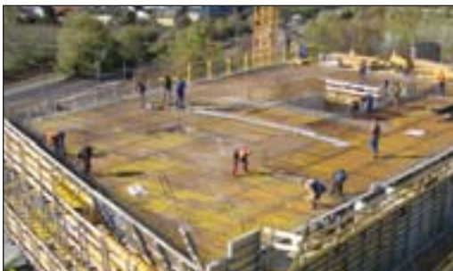
Below, the Vienna Oberlaa Spa project; at the right, construction of the Tauern Spa World.
